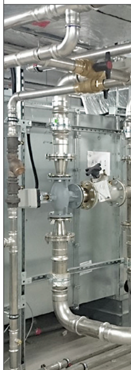
▽ A Geberit Mapress stainless steel pressfit system installed at at the Wellcome Wolfson Institute, Belfast
