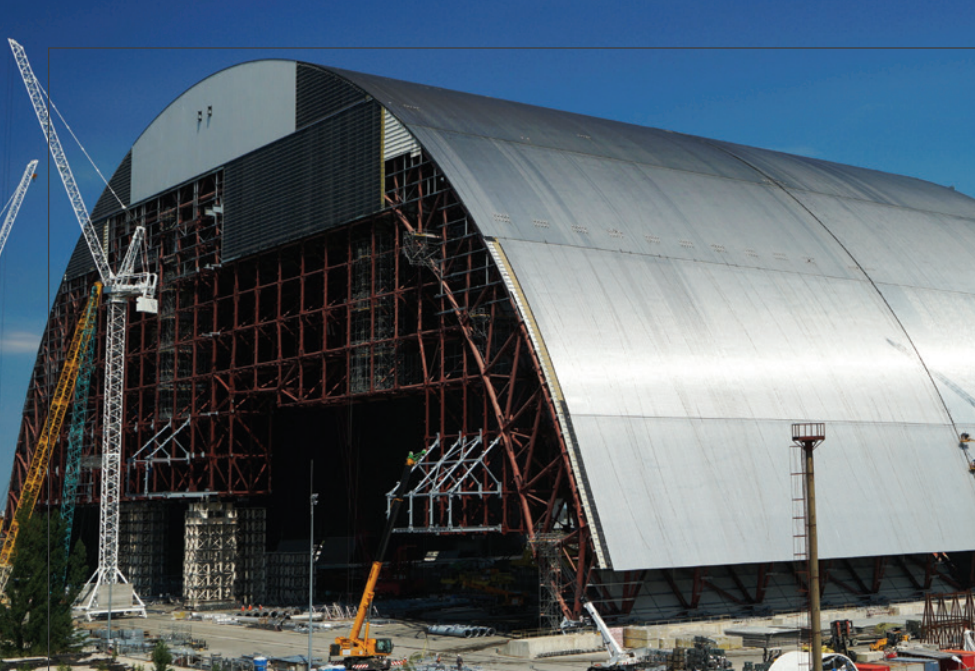
△ The New Safe Confinement shelter has been designed to provide protection for a century or more.
